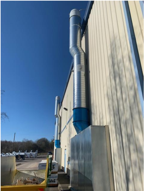
Figure 1.3: Example LEV Extraction Stack (Overseal site)
