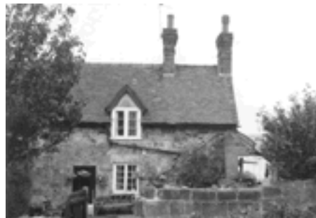
One of the cottages that belonged to the scythe stone workshops. Photographed in 1991. SDDC collection.
