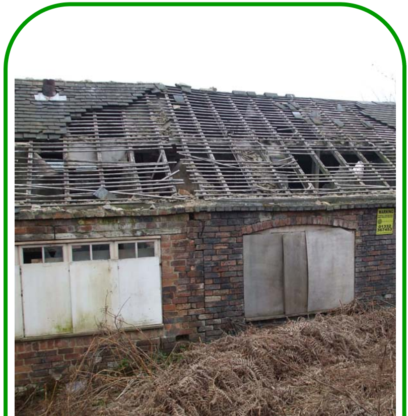
Vandalism and antisocial behaviour are issues in a number of locations in this area
